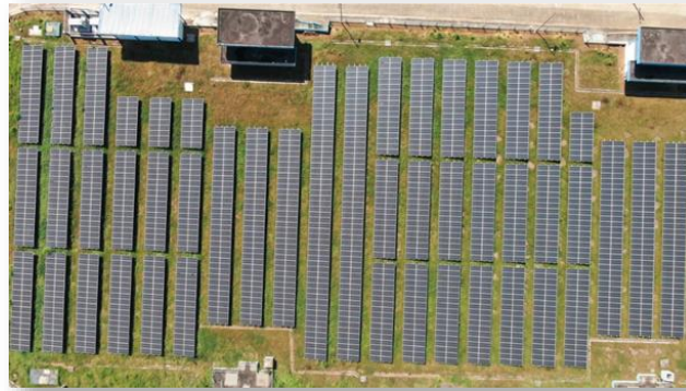
Figure 2. Photo of 1MW Solar Farm
