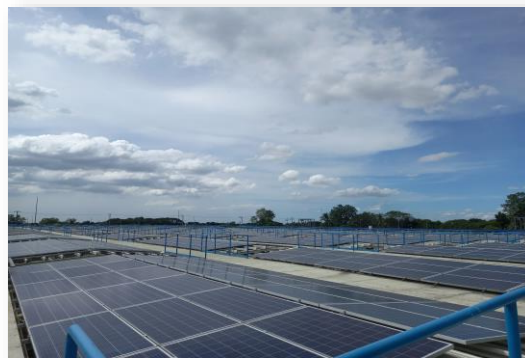
Figure 3. Photo of the 1MW Solar Farm on La Mesa Treatment Plant 1
