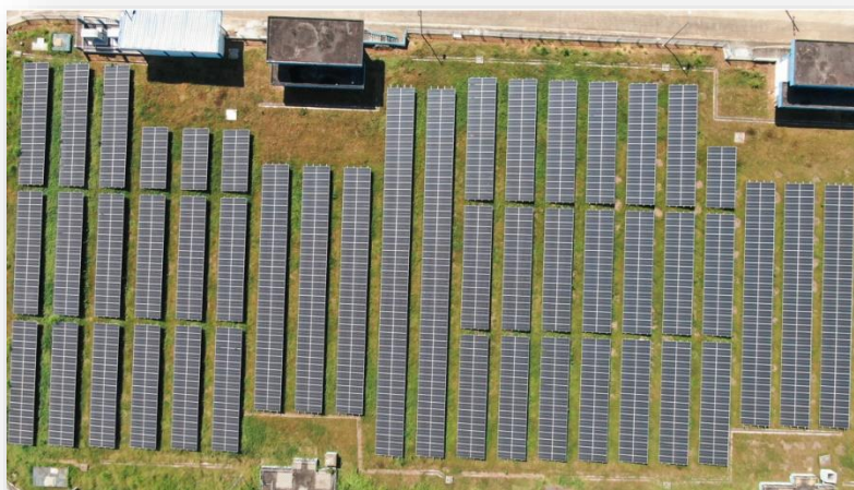
Photo of Maynilad Solar Power Plant (top view)
