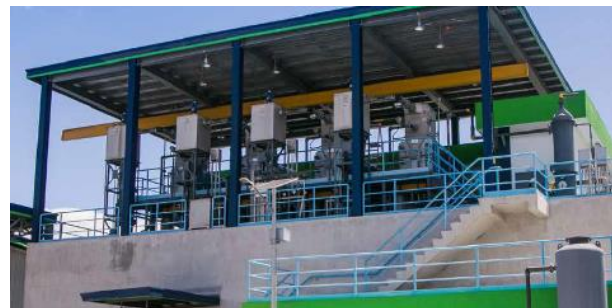
Water Reclamation Facilities, Septage Treatment Plants, Lift Stations and Pump Stations
