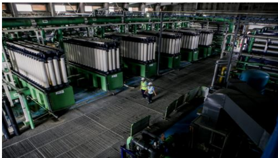
La Mesa Water Treatment Plants 1 & 2, Putatan Water Treatment Plant, Common Purpose Facilities (CPF), Ipo Office Building and Bicti Desilting Basin.
