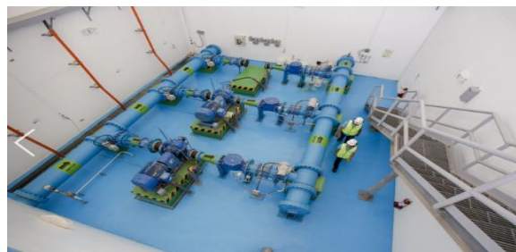
Reservoirs, Pump Stations, Mini Boosters, Deep Well Stations, In-line Boosters and other Special Equipment, Training Facility
