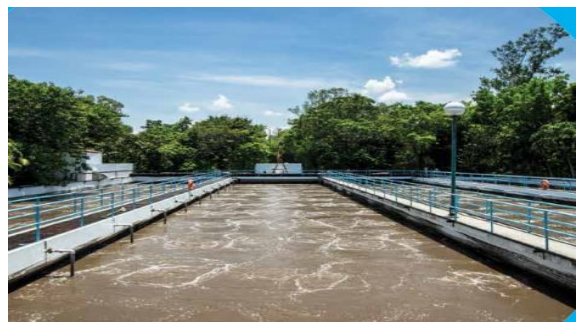
Sewage and Septage Treatment Plants, Sewage Treatment Plants, Lift Stations and Pump Stations and Vitas Desludging Office
