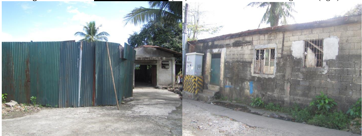
Figure 27. View of [REDACTED] (left) and the condemnable building inside (right).
