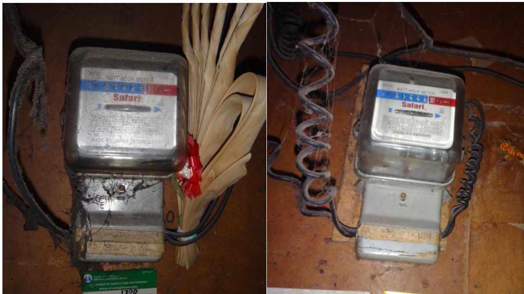
Figure 9. Electric sub-meters installed in each rooms
