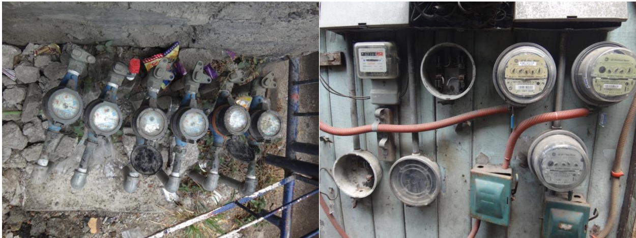
Figure 8. Water and electric meters inside the compound
